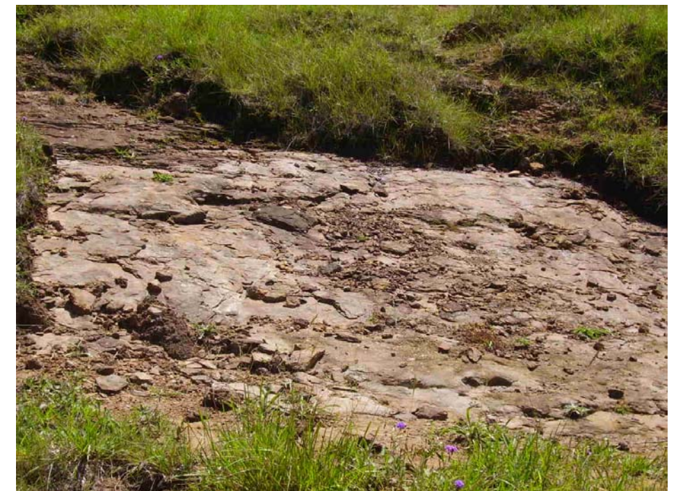
Photo 36F - Instability on Slope along high side of Access Track Zone 2(D). Note shallow depth to rock at this location.
