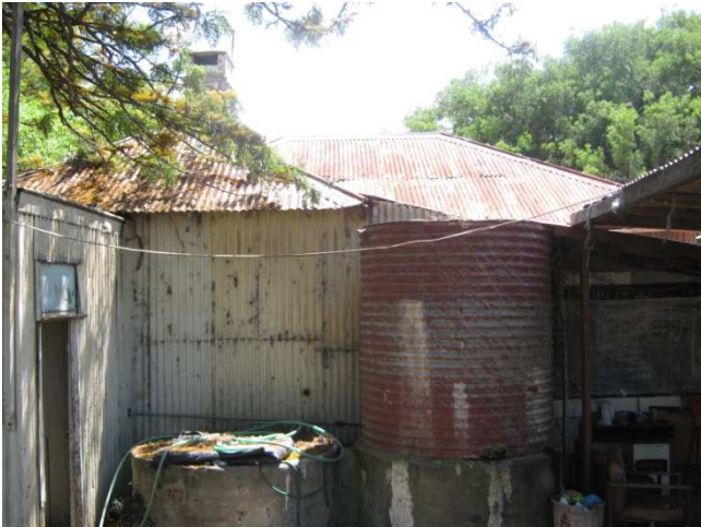
Photograph 5: 01 House, External: Red lead paint to tanks and roof, cream lead paint to walls.
