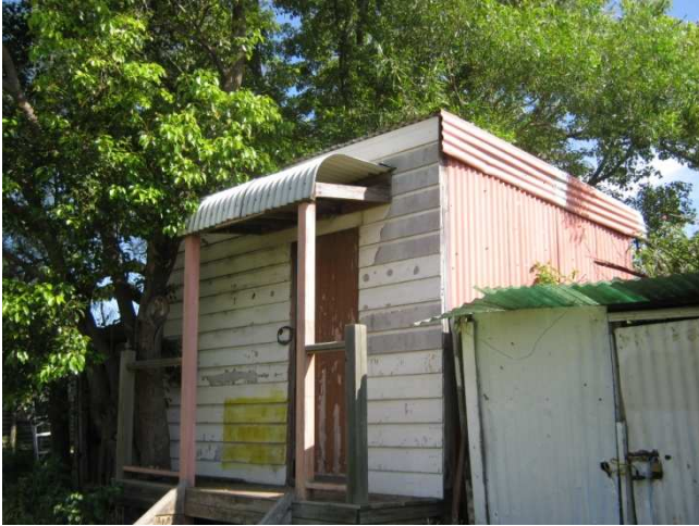
Photograph 31: 16 Shed, External: Red lead paint to roof & side. Locked no access.
