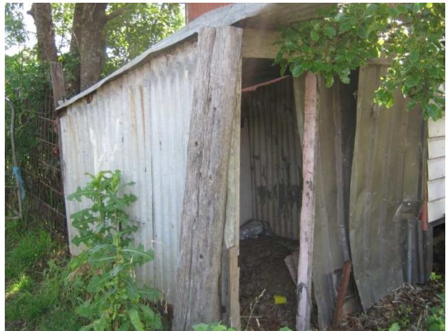
Photograph 30: 15 Chicken Coop, Internal: Cream lead paint to RHS wall.
