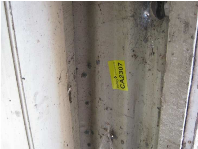
Photograph 3: 01 House, Internal: Car parts store, cream lead paint to walls.
