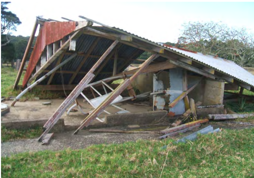
Photo plate 24 - Collapsed structure
