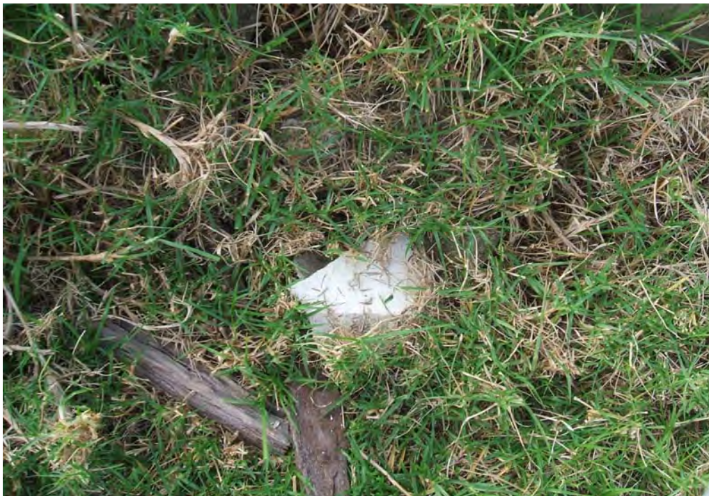
Photo plate 25 - Cement sheeting fragment in grass adjacent to slab
