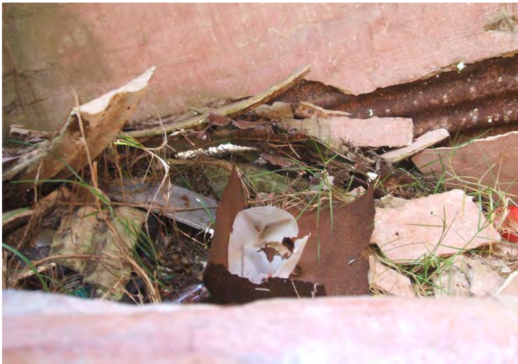
Photo plate 16 - Rubbish inside Corrugated iron tank
