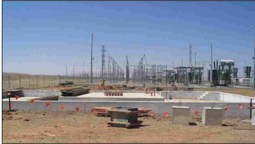
Image 3.10 Transformer foundation (foreground) and electrical substation and switchgear infrastructure (background)
