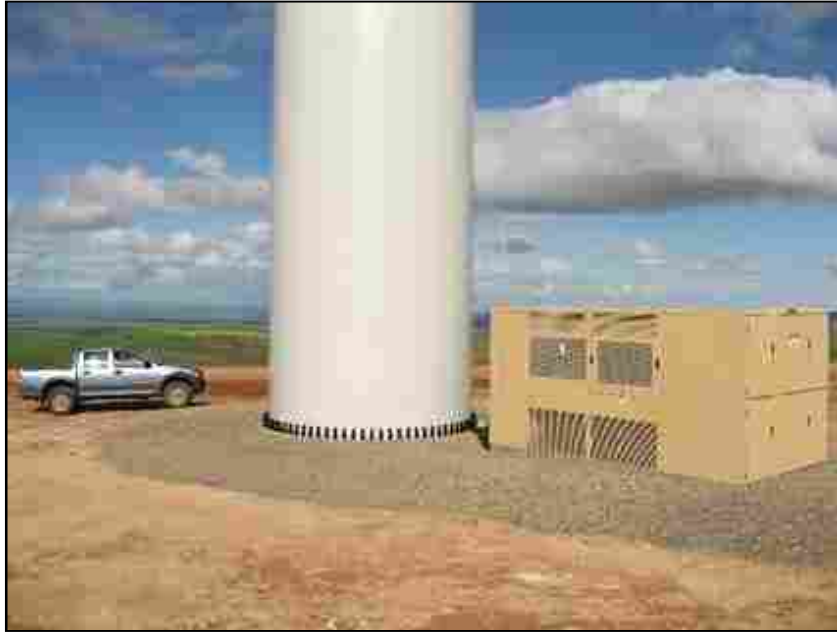
Image 3.5 Transformer adjacent to wind turbine
