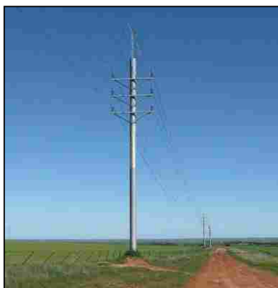
Image 3.6 Double-circuit overhead 33 kV power line
