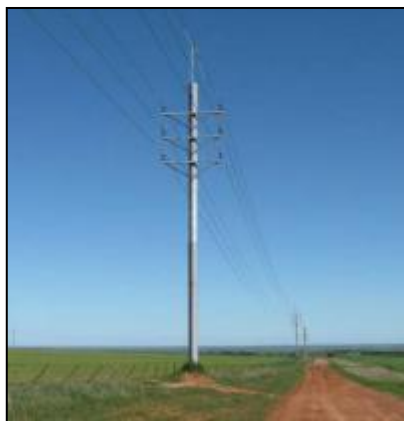
Typical Double-circuit overhead 33 kV power line.
