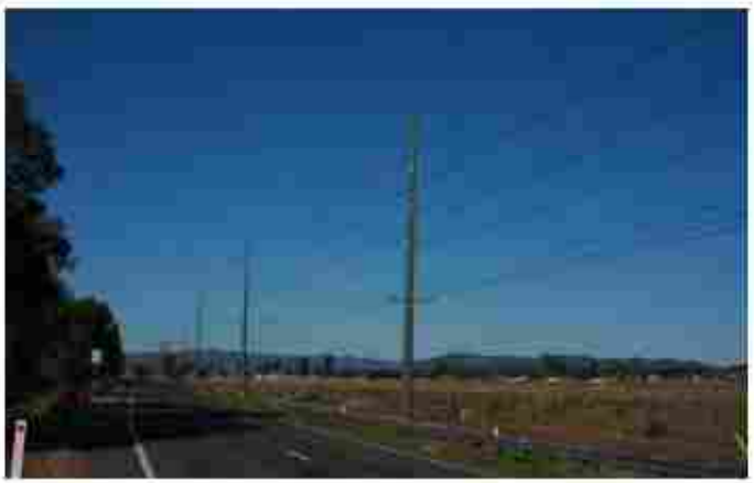
Typical Power Pole
