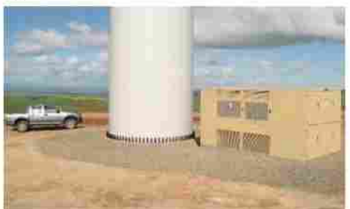
Typical Generator Transformer.
