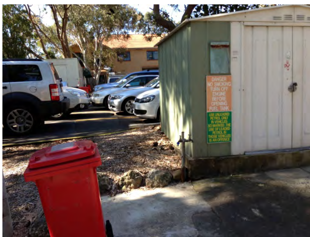
Photo 2 – Danger sign associated with USTs petrol tanks 1 and 2.
