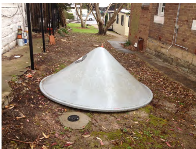
Photo 3 –Groundwater monitoring wells downgradient of USTs.
