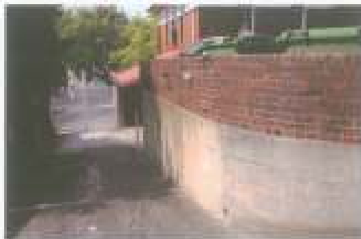
Figure 60 The alleyway down to Butler Street, looking north, with the retaining wall to the right. The wall is in poor condition (Source: Graham Brooks & Associates, July 2006)
