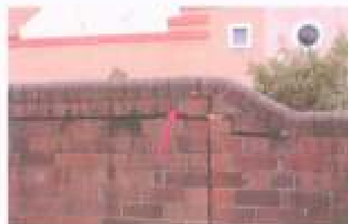
Figure 18: The state of repair on the perimeter wall is at some points quite poor and sections built on the support further additions over time. (Source: Graham Brooks & Associates, July 2006)
