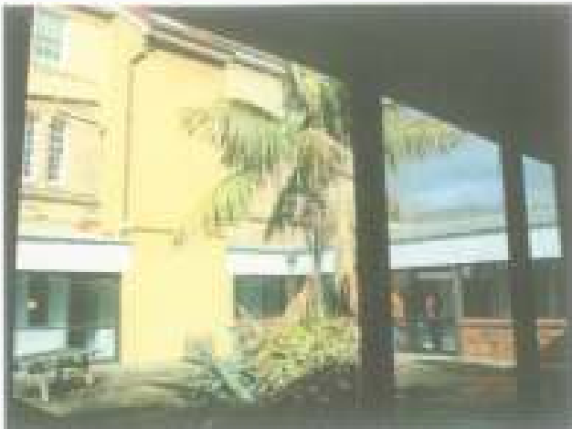
Figure 54: Exterior courtyard looking towards main building. The view shows the many changes by modern and adaptations of the complex. The third floor addition is seen, making comparisons, modern masonry work, aluminium window components and plumbing installations.
