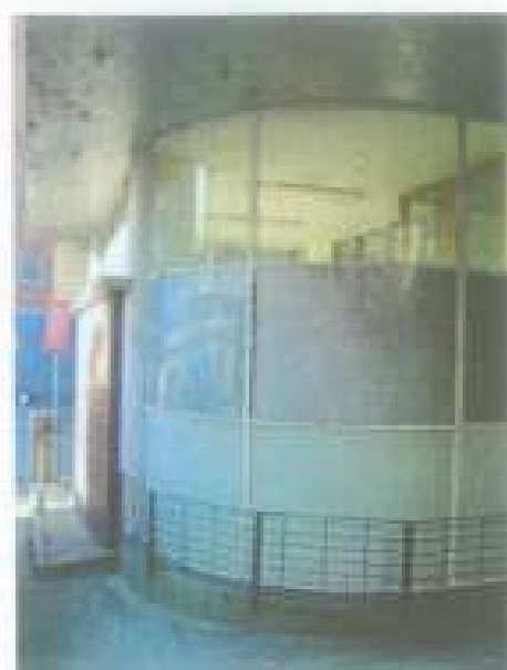
Figure 26 An image taken at the former entrance area to the subject building, the former Outpatients Block, and now the Cohen Wing, showing evidence of deterioration of finish on steel frames and concrete, how the modernist curved glass surface, the slender concrete column work, and the horizontally oriented window openings. (Source: Graham Brooks & Associates, July 2008)
