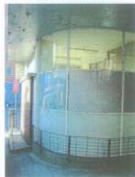
Figure 16: Front entrance way of the O'Brien Wing, showing signs of deterioration, but characterised by the clean horizontal lines and gleamed stone of the modern wing design. (Source: Graham Brooks & Associates, July 2008)
