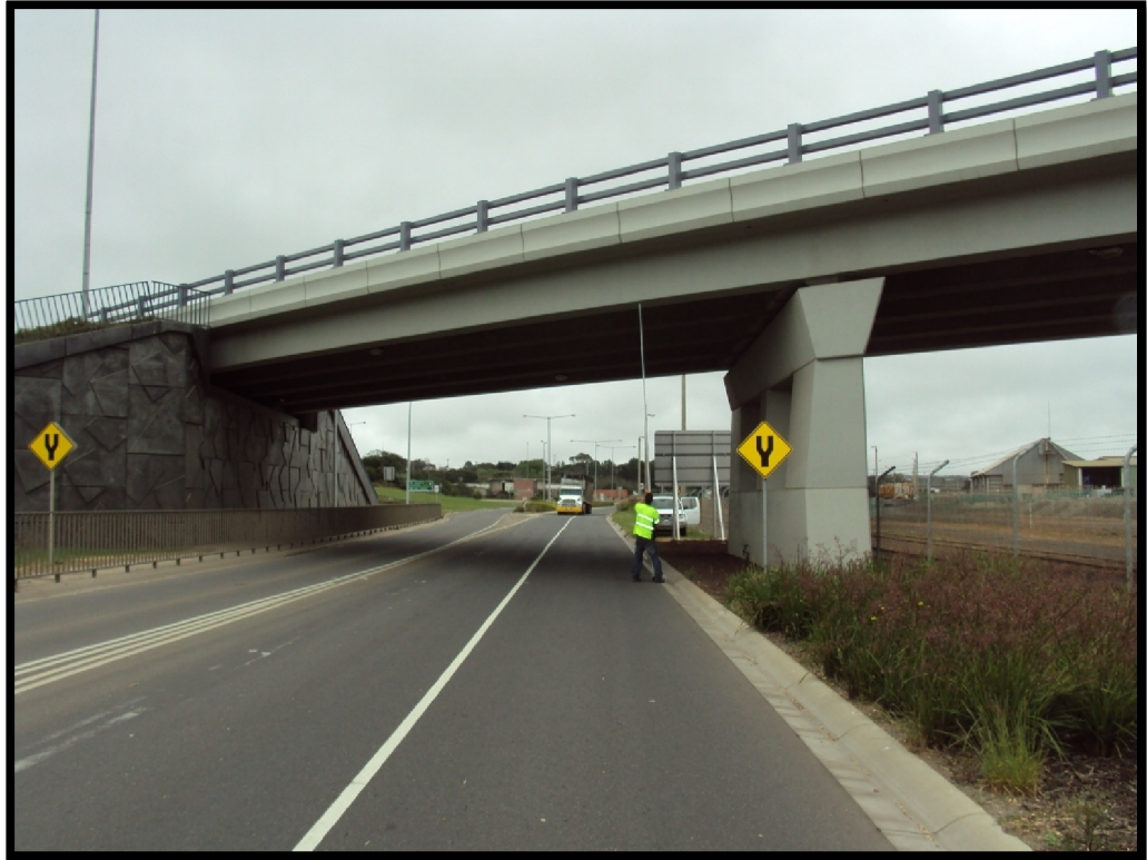
Figure 5.3: Identification of bridge underpass height risk
