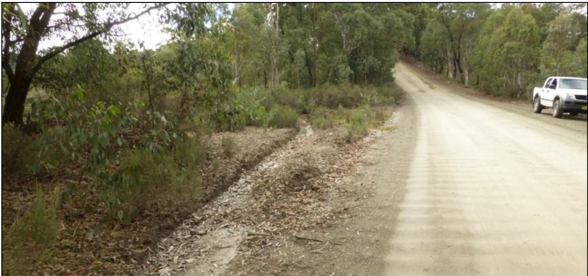
Grade 2: RHS - Clearance and levelling required, on straight section of road.
