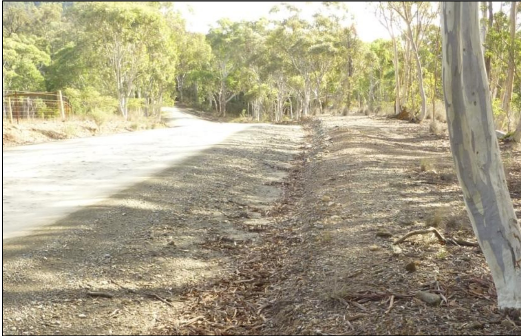
Grade 3: RHS - Levelling required, not a wide roadside area. On a slight bend.
