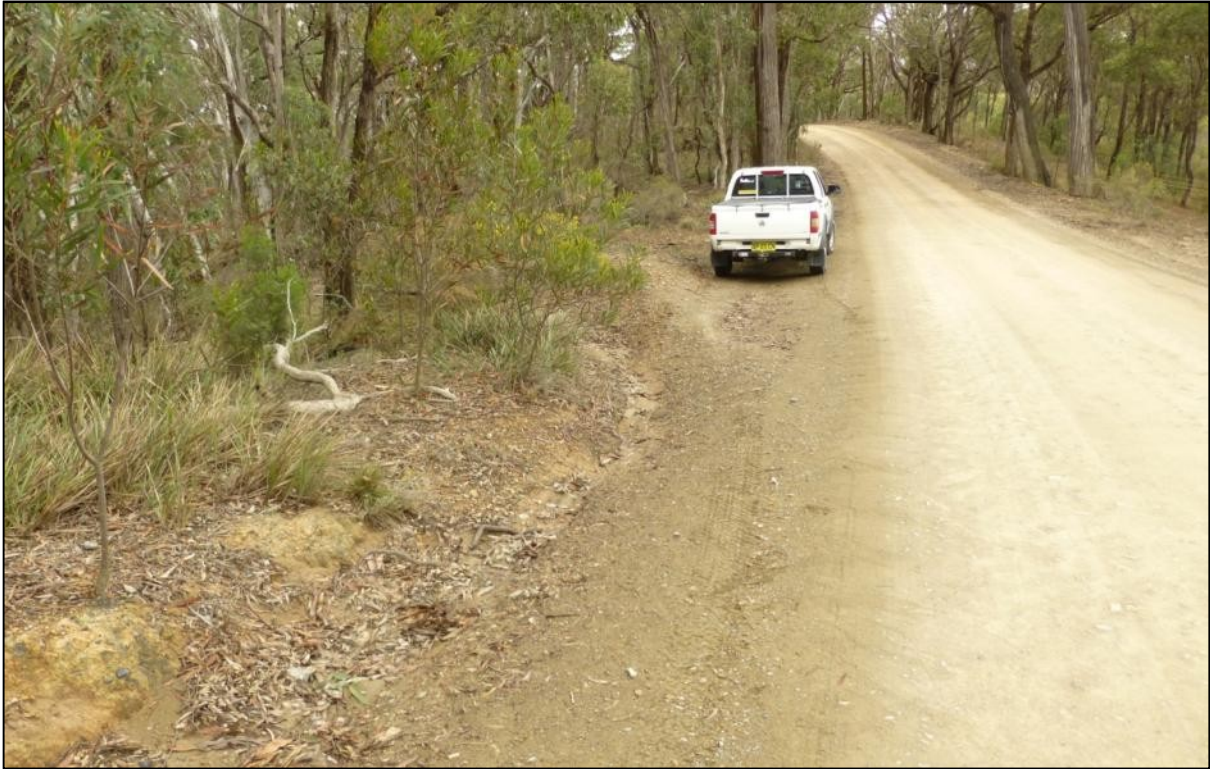
Grade 3: LHS - Located opposite a driveway. Clearance and levelling required, straight section of road.
