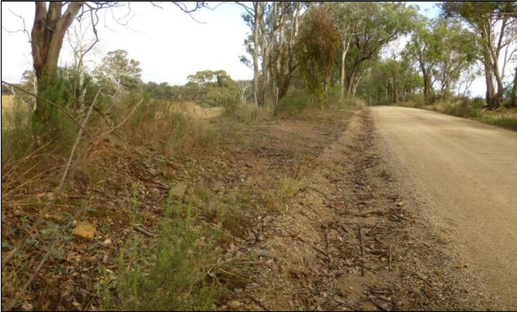
Grade 2: LHS - Would require some clearing and levelling, straight section of road.
