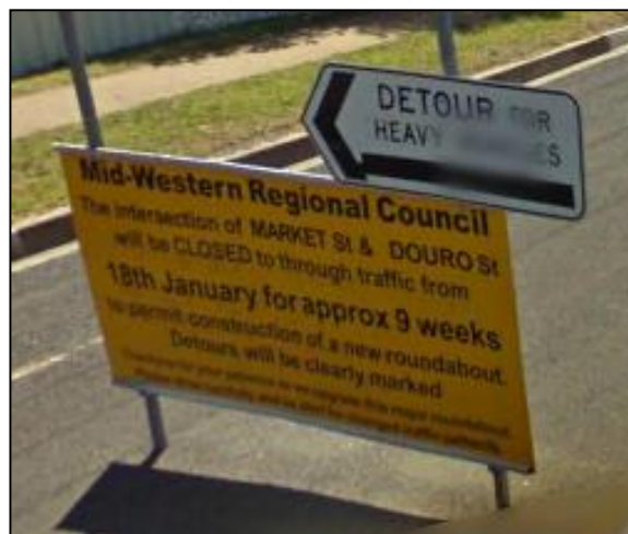
Figure 2 Image of a heavy vehicle detour sign used during the upgrade of the Market Street / Douro Street roundabout. This signage directed heavy vehicles to detour along Cox, Short and Lewis Streets (image courtesy of Google maps).
