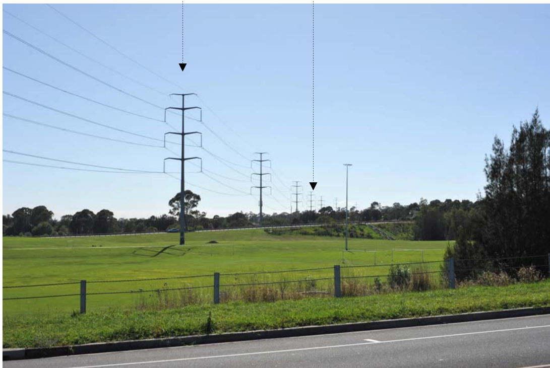
Plate 16 Existing 330 kV double circuit powerline
