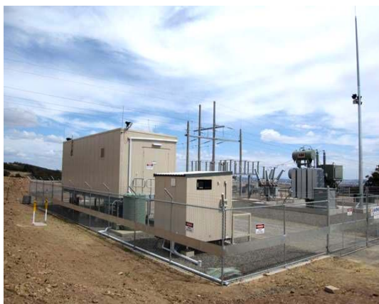
Plate 11 – Typical wind farm collector substation
