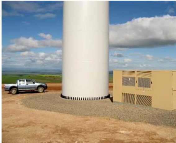
Plate 13 – Typical of a generator transformer
