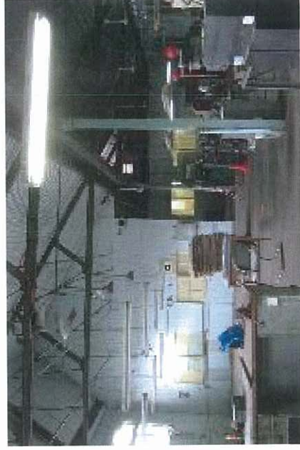
Telecommunications Building - Interior
