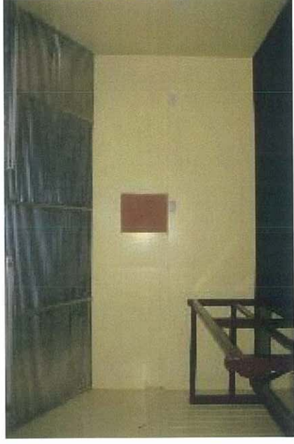
Telecommunication Building - Mezzanine
