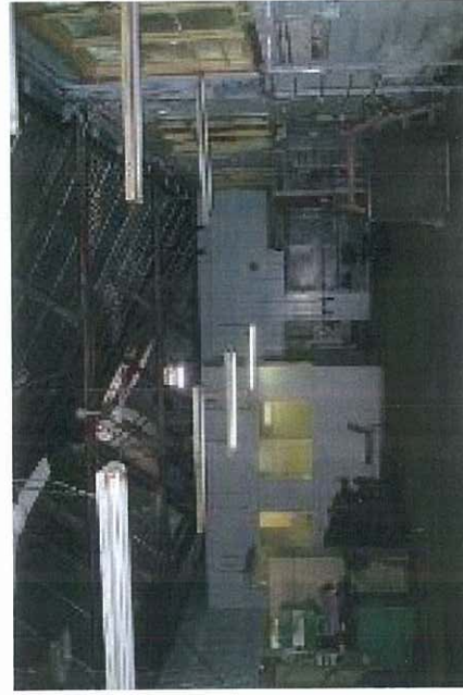
Telecommunications Building - Interior
