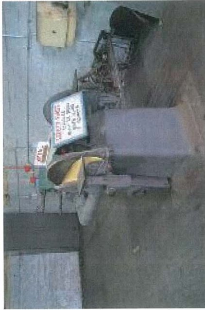
Telecommunications Building - Interior
