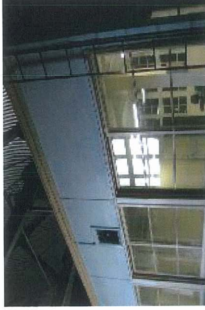
Telecommunications Building - Interior
