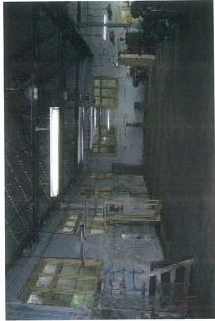
Telecommunications Building - Interior
