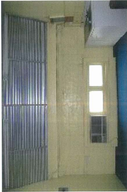
Telecommunications Building - Interior Mezzanine
