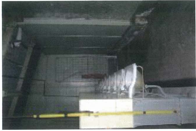
Telecommunications Building - Interior
