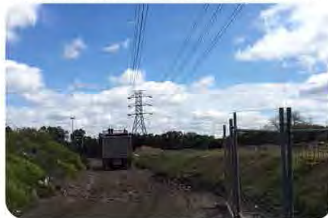
Existing power lines
