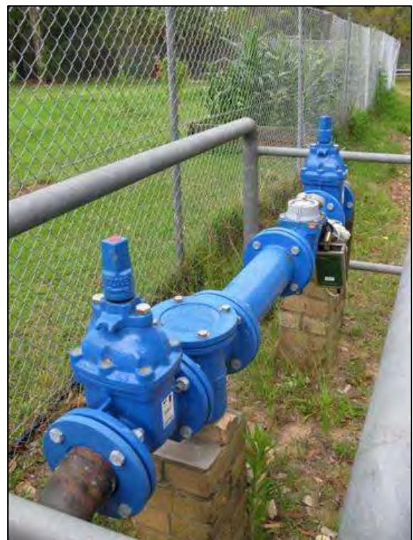
Figure 4. Sports Fields Main Meter
