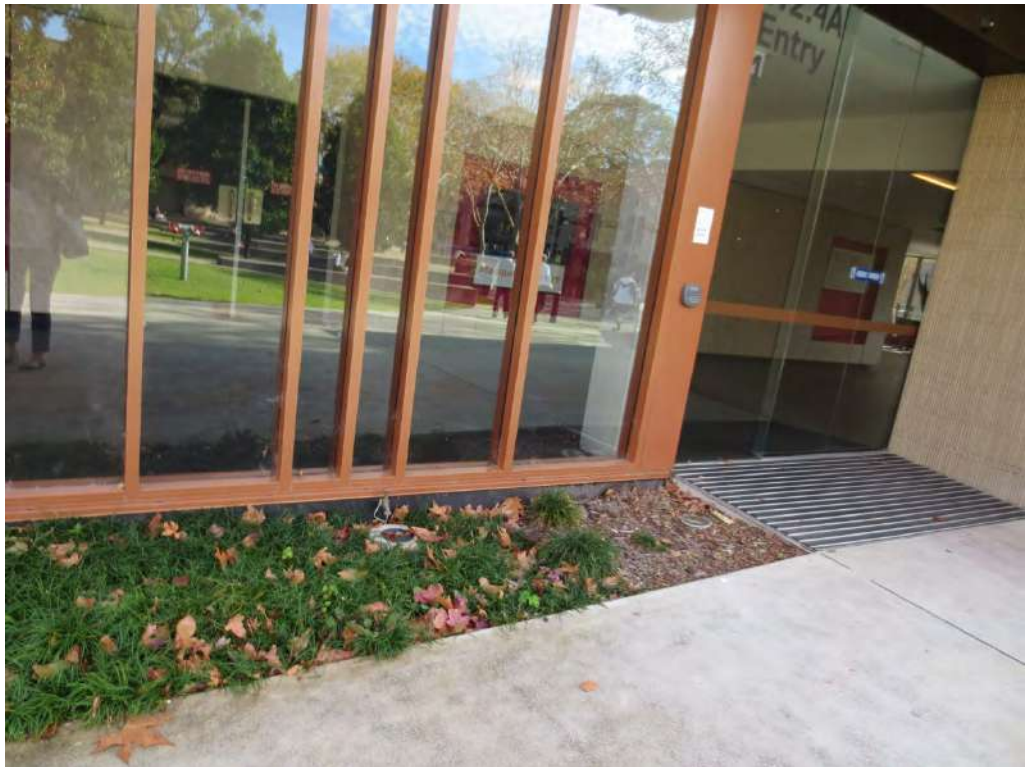
Figure 38 Mondo Grass bed requiring replacement planting
