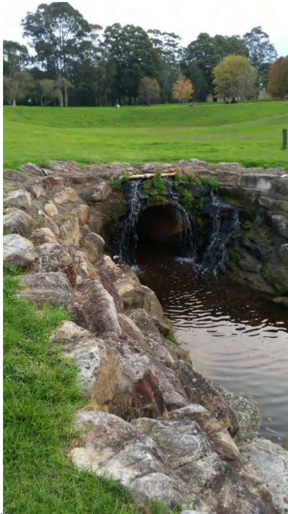
Figure 10 Underground culverts on Mars Creek should be considered for removal. This pipe travels in a direct line under the amphitheatre so the creek may need a slight diversion if the pipe is removed. Note that very little water is actually flowing in the pipe.
