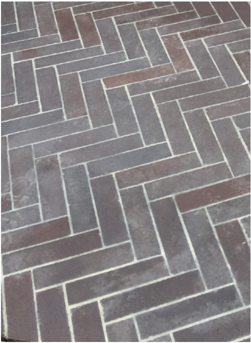
Brick paving, Herringbone - Kensington Street
