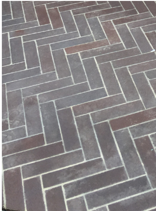
Brick paving, Herringbone - Kensington Street
