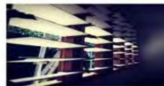
LOUVRES Louvres for cross ventilation
