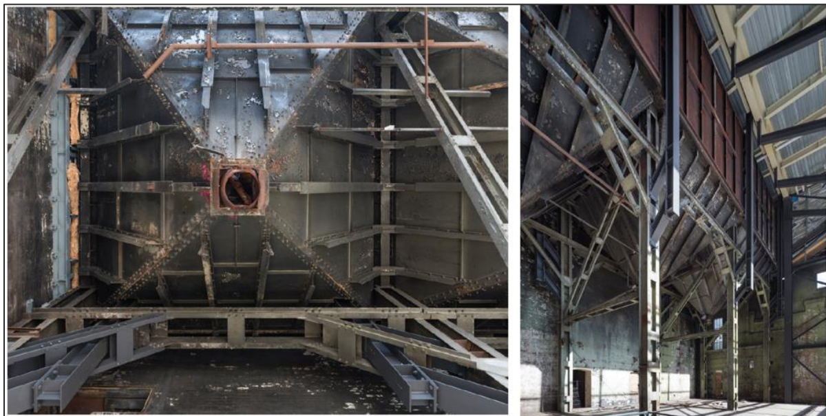
Figure 12 | View of the three existing coal hoppers in Building 30 (Source: RRF1 2 Attachment 1 - Hopper Removal Study)
