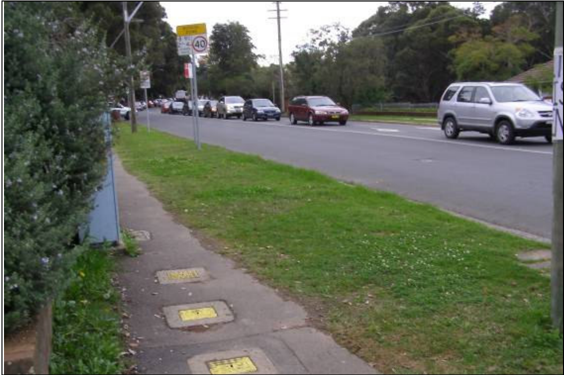
Photograph B.005 - Gas main in Fox Valley Road verge-
