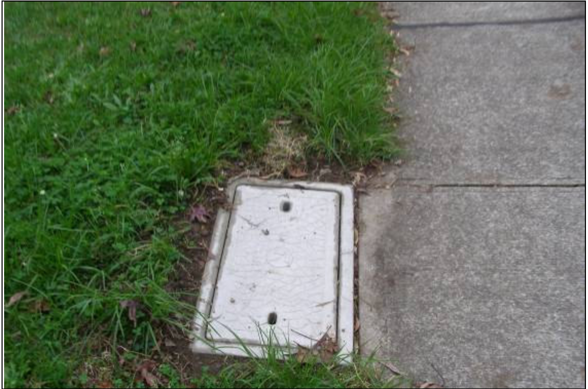
Photograph B.003 - Telecommunications in Fox Valley Road verge-
