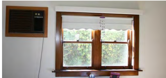
175 Fox Valley Road window and new air-conditioning system
