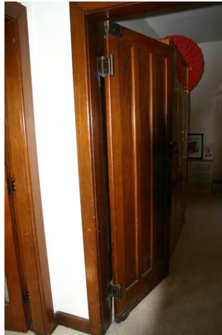
175 Fox Valley Road dining room door. Note kick plate adjacent to lower hinge
