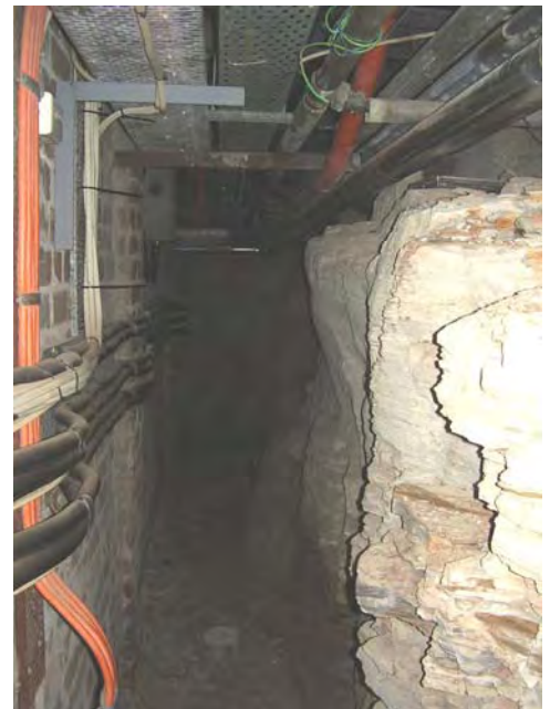
Photo 3: The footing access area for the basement of Building 4. Note the shale located immediately beneath the footings and other service pipes/cables
