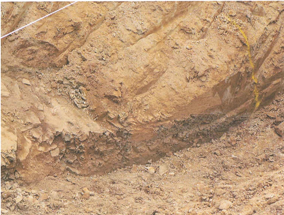
Plate TF4. Chn.17m to 22m. Fault plane dipping (downstream) into the floor of the trench.
