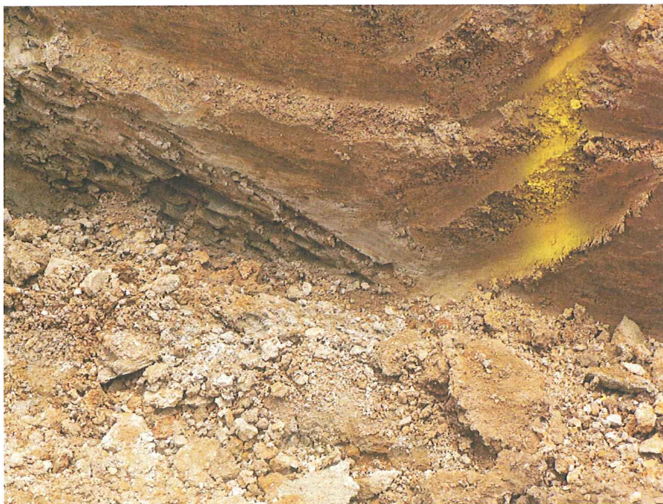
Plate TF10. Fault plane dipping into the floor of the trench.
