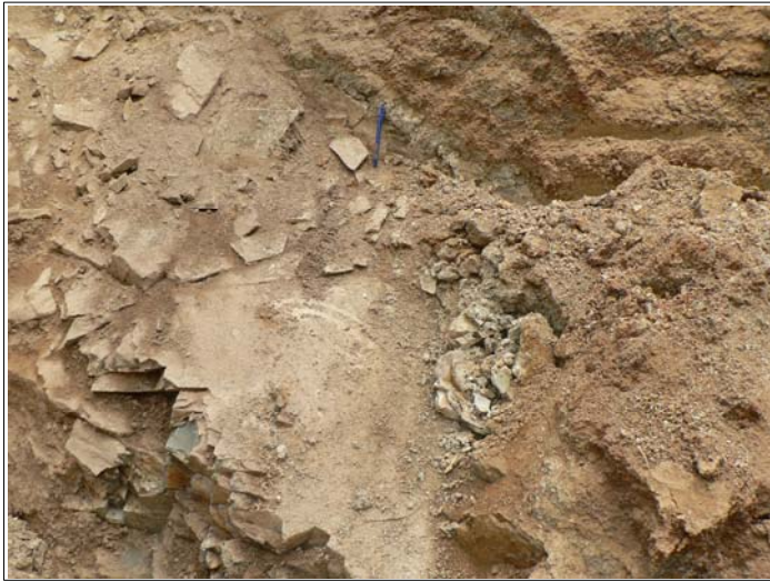
TF7 – Fault plane dipping downstream
