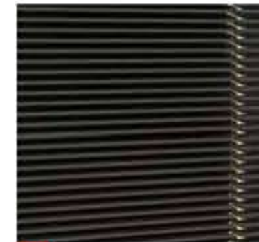
SUBSTATION METAL LOUVRE SCREEN
