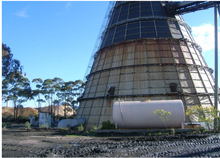
Plate 13-1 View of Burner and Fuel Storage Tank
