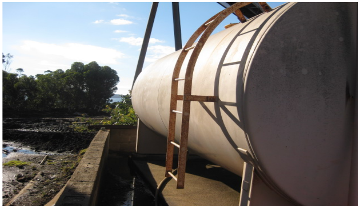
Plate 13-2 View of Fuel Storage Tank in Concrete Bund
