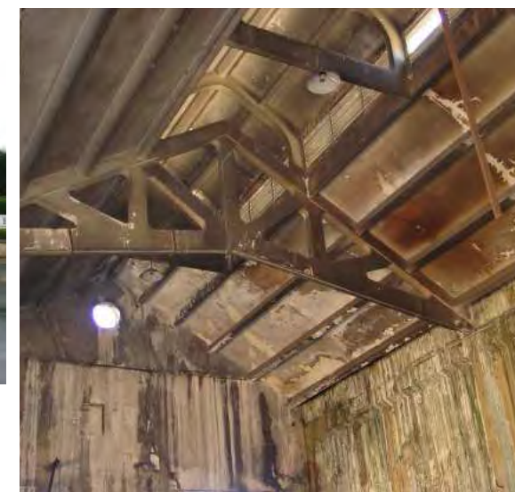
The Powehouse - Interior
