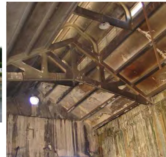
The Powehouse - Interior
