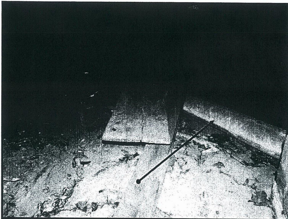
Photograph 5: Bambi Kindergarten, under-croft – asbestos cement debris (Refer to sample Bam/08)
