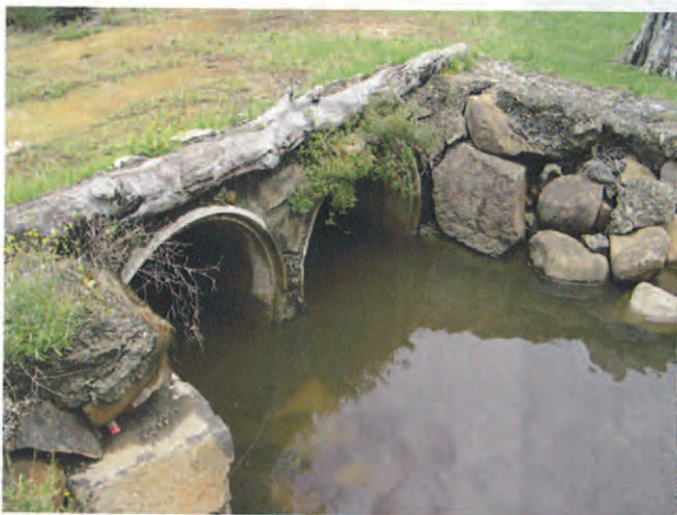
Figure 6: Tidal floodgate on Dunn's Drain
