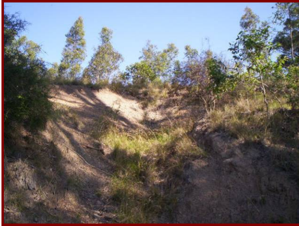
Photo 34 – Slumping/erosion of slopes on Western side
