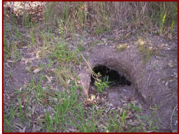
Photo 35 – Piping erosion of slope
