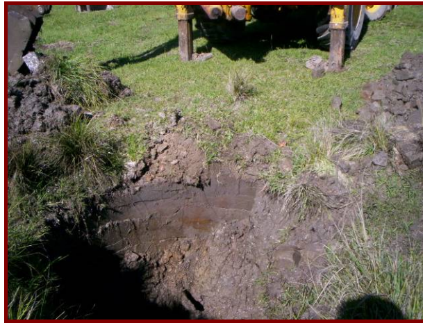
Brick Cistern at Reported Location of Pothole P7
