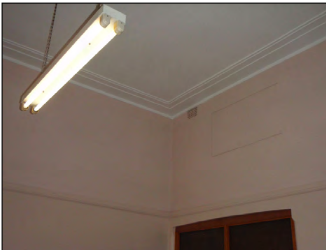
Figure 96: Ceiling detail in 1946 section. In other areas, the original ceilings have been replaced or covered over.
