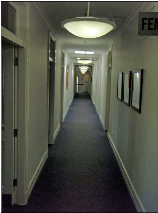
Figure 154: First floor hallway, showing rooms to either side with profiled timber skirting, simply profile cornices and doors with top lights.
