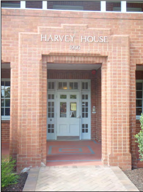
Figure 147: Detail of the entrance porch. The tiling is of a later period. The Art Deco Style detailing of this porch stands in marked contrast to the otherwise Interwar Free Classical of the building and looks forward towards the Functionalist Style (a development of the Art Deco Style) that was soon to dominate hospital architecture.
