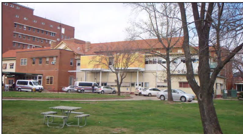
Figure 84: The northern elevation of the 1922 wing, enclosed by fibro-clad walls, with recent service pods and air conditioning units.
