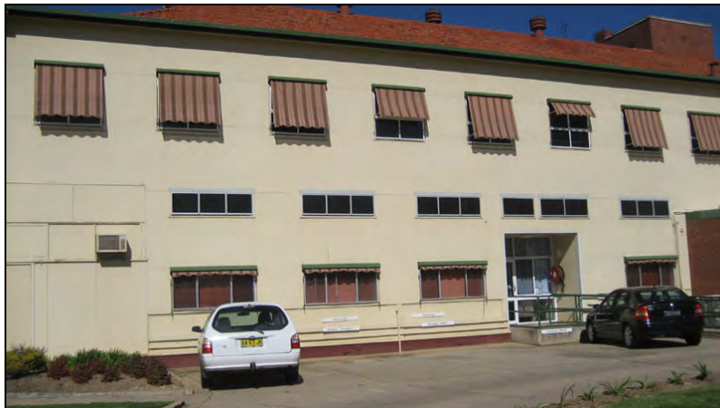
Figure 81: Northern elevation of the original 1910 wing, now enclosed in fibro clad stud walls.
