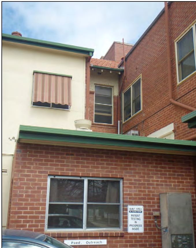
Figure 88: An original double hung window (top centre) in the 1910 building, with the head set into the upper rough cast band and a fine brick sill detail. This photograph also shows typical alterations to the 1946 addition, being the replacement of timber framed double hung windows with aluminium-framed windows. Note also the proliferation of services that characterise this elevation and the roof of the Old Building.
