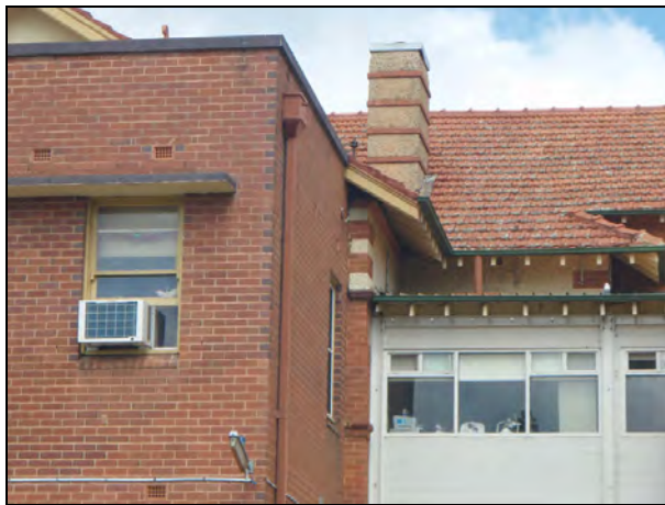
Figure 86: Detail of an original brick banded chimney, the top of which has been removed and capped. Note also the exposed timber rafters.
