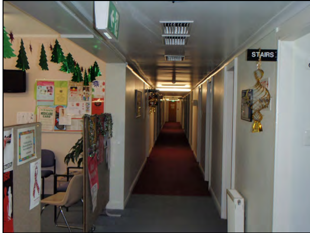
Figure 139: Typical hallway in Lewis House, showing rooms leading off either side of a narrow corridor. Note the simple cornice and skirting detail.
