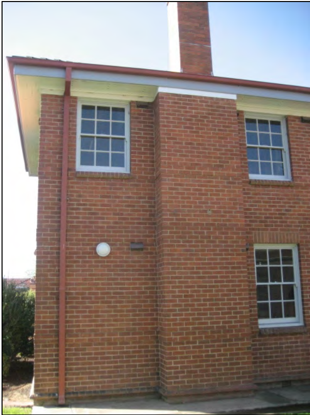
Figure 149: Detail of the southern elevation, showing closed eaves, chimney breast and multi-pane windows.
