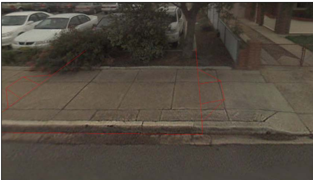
Figure 4.3.1 – Broken Kerb/ Footpath on Northern Side of Yabtree Street
