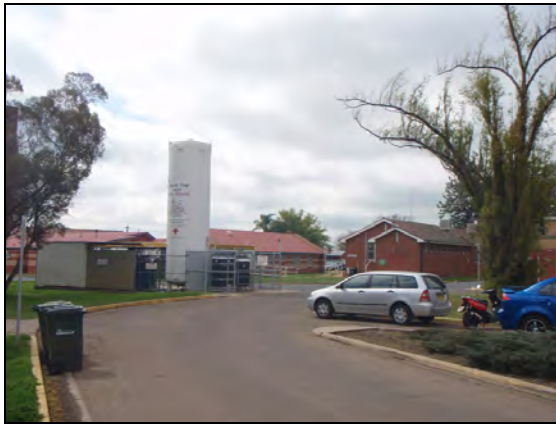
Figure 129: Flammable Liquid Stores and Medical Gases Compound.
