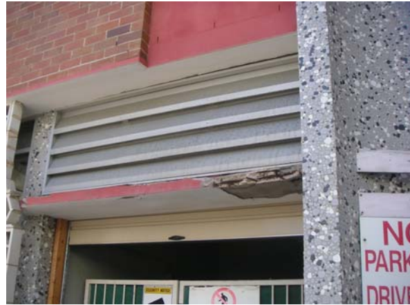
Example of deterioration of built fabric
