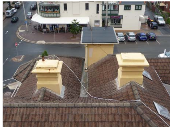
Detail of terrace roof showing project bay (left) and tower element (centre) with central chimneys
