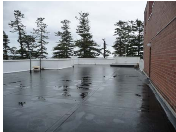
Roof, looking east (right roof top building is on 1970s Norman Drummond Building)
