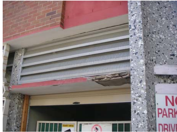
Example of deterioration of built fabric
