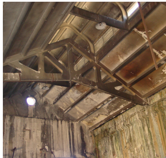
The Powehouse - Interior
