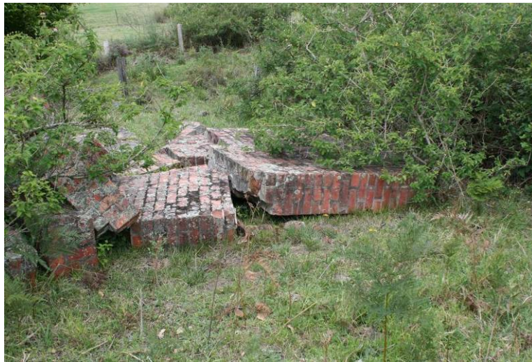
Photograph 5.22 View of collapse tank stand piers (ERM 2007)
