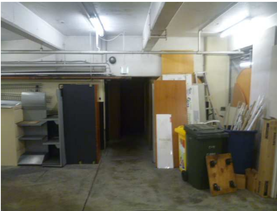
Figure 4.5 Level Two basement, showing doorway with two areas that were inaccessible during the site inspection, the pump sump and the boarded off area. (Source: GML, 2010)
