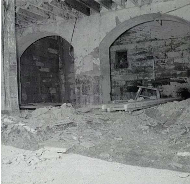
Figure 4.1 Photograph of sandstone vaulted archways under Macquarie Street, 1964 appears to show demolition in process. (Source: City of Sydney Archives, Citation: NSCA CRS 48/3825).
