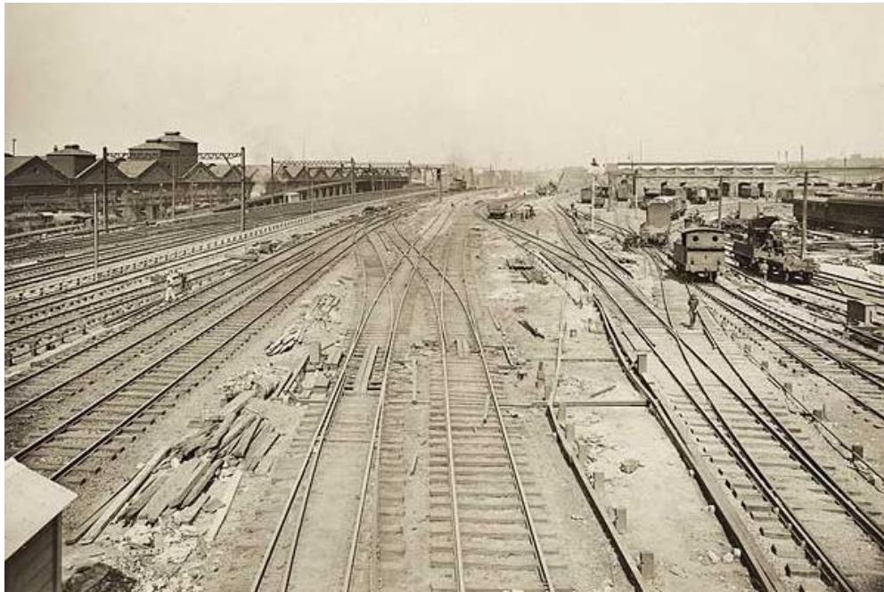
Figure 8 - Illawarra Steam Dive under construction - view from Workmen's Footbridge Eveleigh looking west, undated. Source: 877/33, State Records
