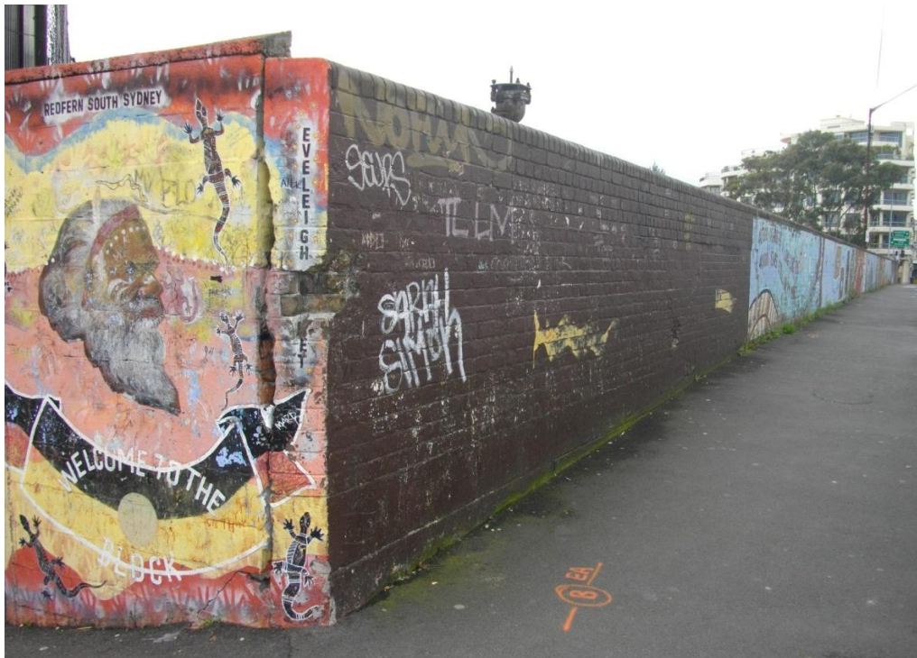
Figure 26 – View of the corner, showing the junction of the English bond brick wall to Lawson Street (right) and the mural painted concrete block wall to Eveleigh Street (left) (Source: NBRSPARTNERS, June 2011)
