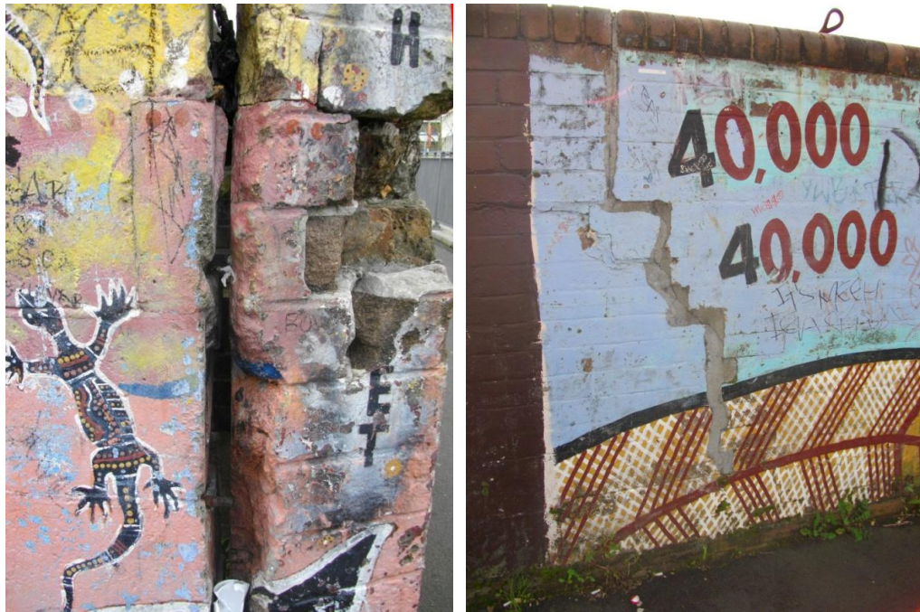
Figure 27 – Detail of the corner junction, showing the fractured “9-inch” English bond brick wall at the corner to Lawson Street part of the original wall constructed in 1891 (left). Lawson Street railway wall showing the repaired structural cracking near the junction of the original wall and the later addition wall, added as part of the widening of the railway corridor (left). (Source: NBRSPARTNERS, June 2011)
