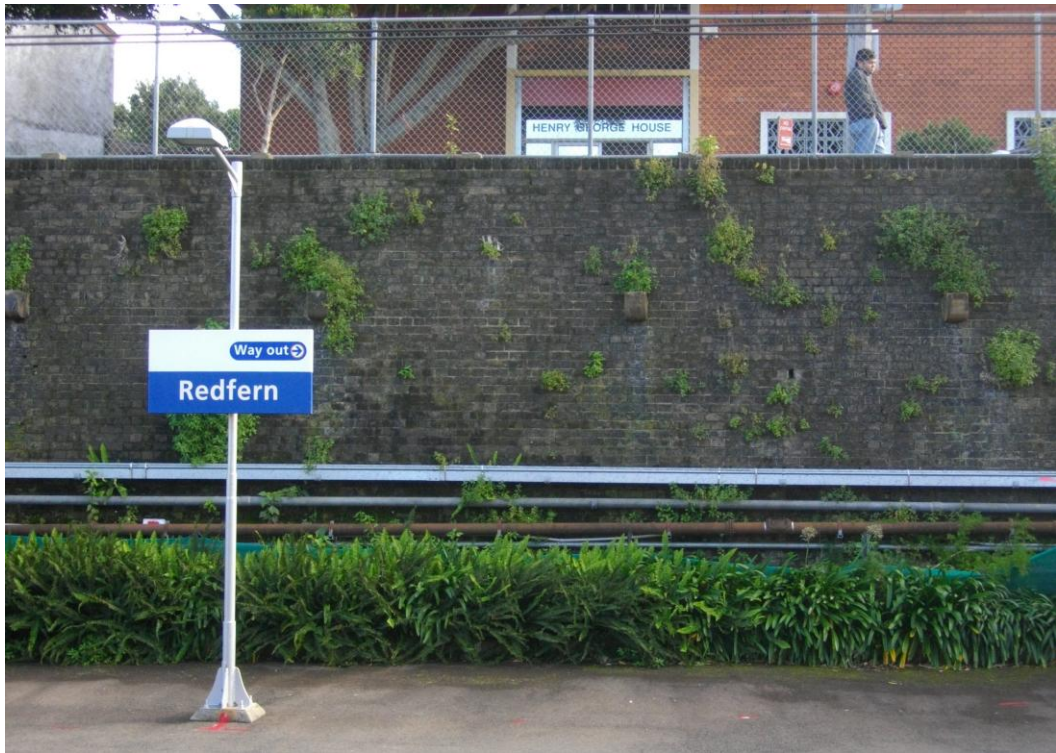
Figure 21 – View north to the brick retaining wall along Platform 1 at Redfern Railway Station. This retaining wall appears to be the same construction as the railway corridor on the retaining wall to the north (Source: NBRSPARTNERS, July 2011)
