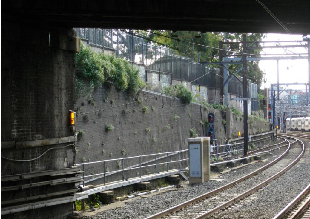
Figure 18 – View north from Platform 3, Redfern Railway Station, to the rail corridor retaining wall. The retaining wall is constructed of facebricks in English bond, possibly around 1885-1891. Engaged piers provide support for the overhead wiring structures introduced when the rail line was electrified from 1926. A stepped blockwork fence / wall with metal palisade fence above and stepped back from the railway corridor retaining wall. Recent overhead wiring structures have been installed on top of the retaining wall (Source: NBRS+PARTNERS, July 2011)
