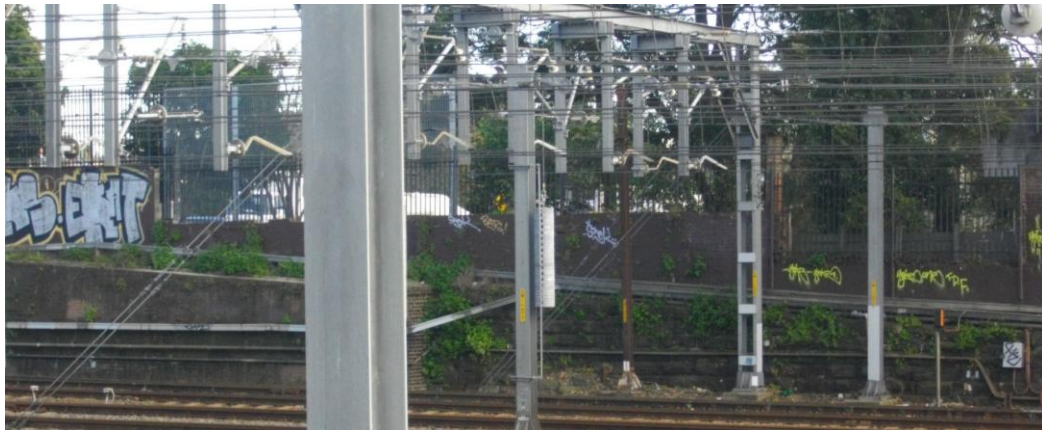
Figure 20 – View west from Gibbons Street across the tracks showing the junction of the brick retaining wall and sandstone retaining wall to the north (at right) (Source: NBRS+PARTNERS, July 2011)
