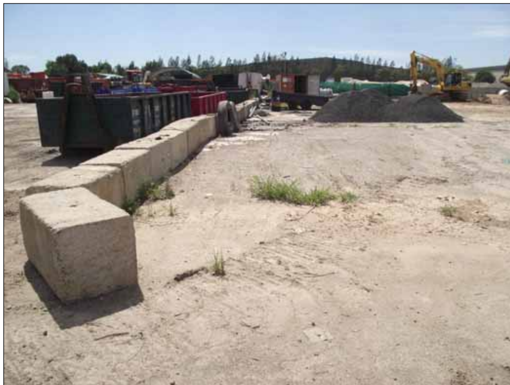
Plate 1: Construction material stockpiles, concrete blocks and metal containers located in the west survey area.
