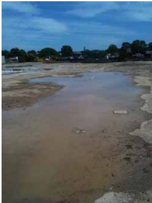
Figure 2. Large puddles of water in Area 1.
