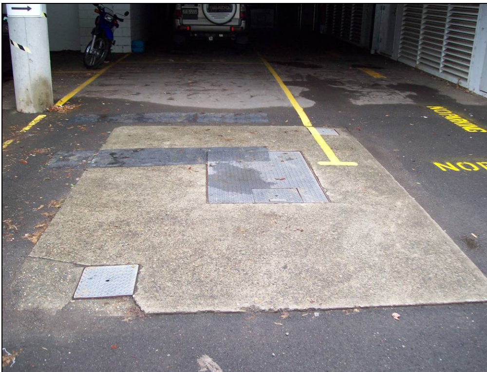
Photo 4 – Underground fuel storage tank to the east of the proposed western building envelope
