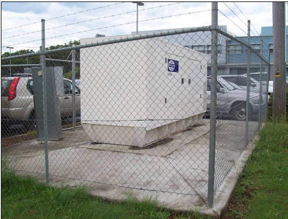
Photo 13 – Emergency generator in the proposed eastern car park area
