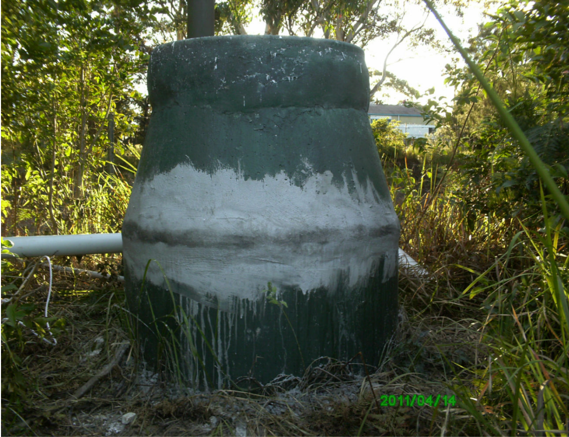
Photo 41-Sewer rising main manhole and vent pipe
