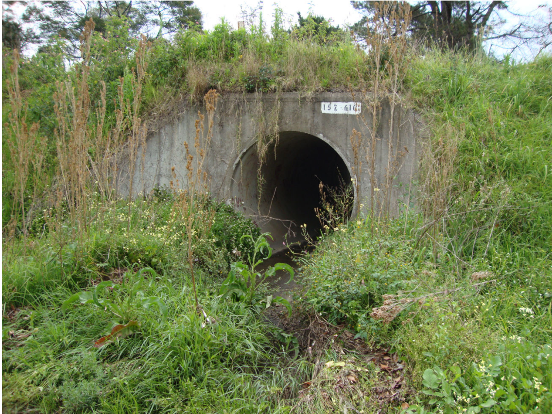
Photo 46b- Large pipe culvert in rail reserve on west side of Railway Street
