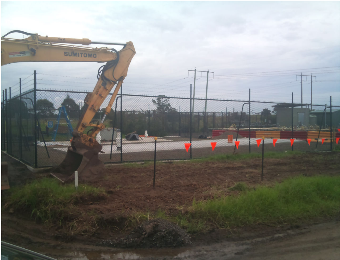
Photo 1- Eastern Gas Pipeline tie-in point at Pestells Lane (valve and meter station)
