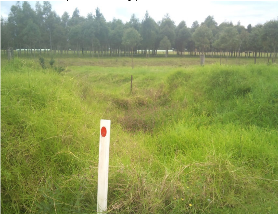
Photo 18- Example of tail-out drains on south side of Fletchers Lane, leading into Open channel drain
