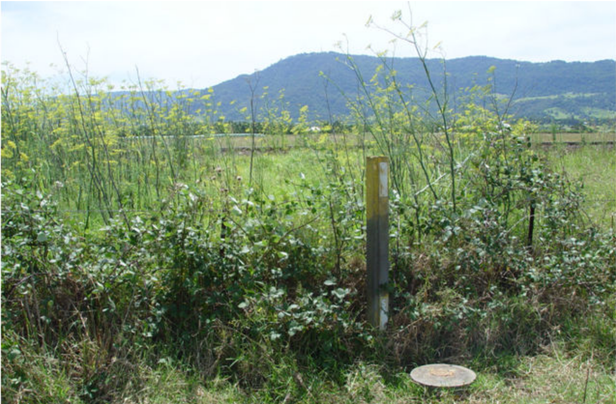
Figure 18: Water main infrastructure within road reserve, between waterway crossing 1 and waterway crossing 2
