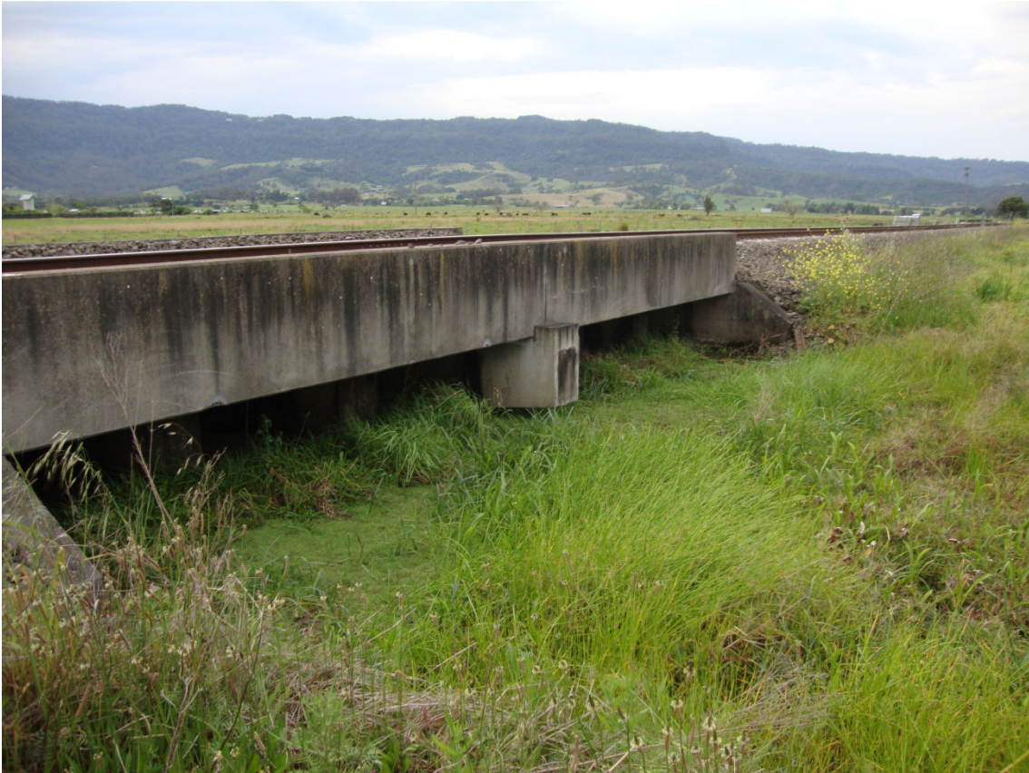
Photo 25a-Culvert between first and second waterway crossings for low lying area in rail reserve, adjacent to road reserve
