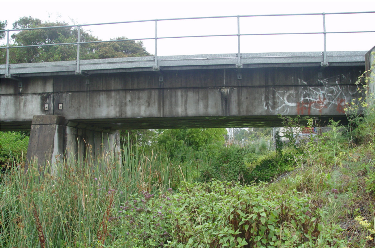
Figure 32: Heavy weed infestation at waterway 4 crossing
