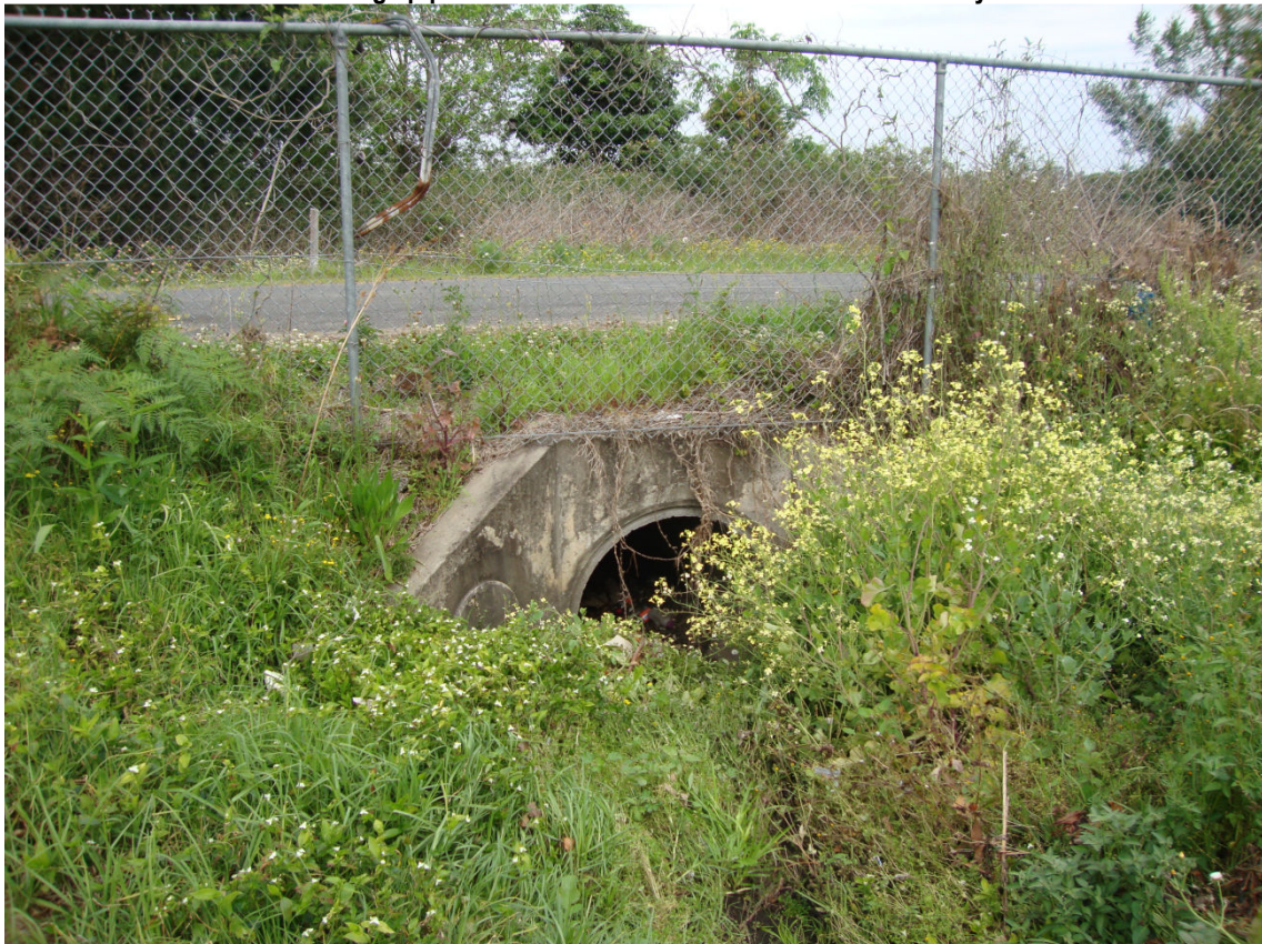
Photo 46c- Small headwall for pipe culvert under Railway Street, taking stormwater from large pipe culvert shown in previous photo.
