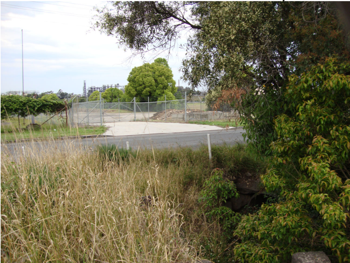
Photo 53b- Stormwater infrastructure under road reserve beginning on west side of Railway Street, leading into pit on east, shown in following photo 53c
