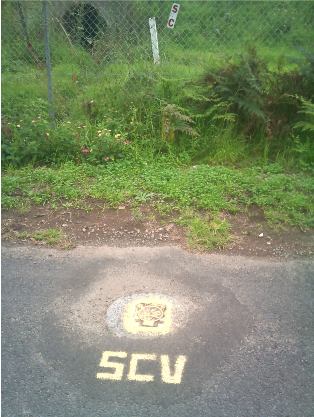
Photo 46a- Scour valve shown with Large pipe culvert in background leading into drainage system under Railway Street
