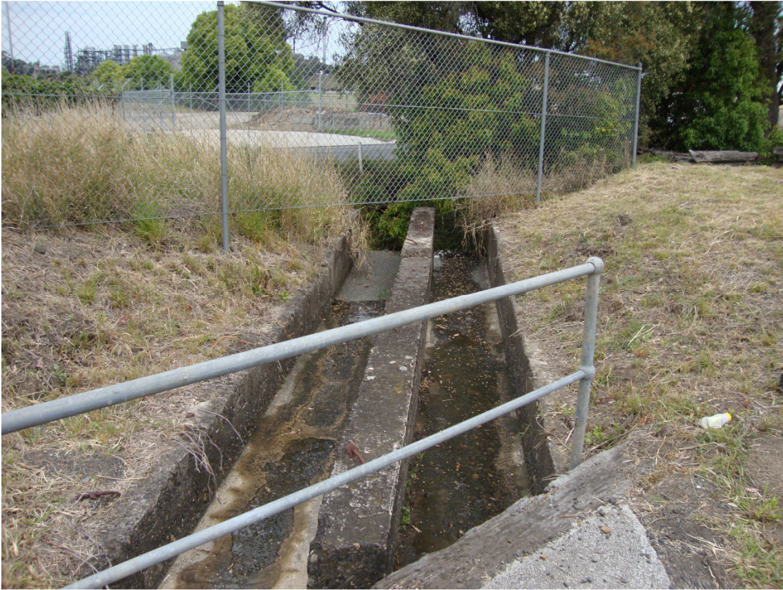
Photo 53a- Stormwater infrastructure in rail reserve on west side of Railway Street
