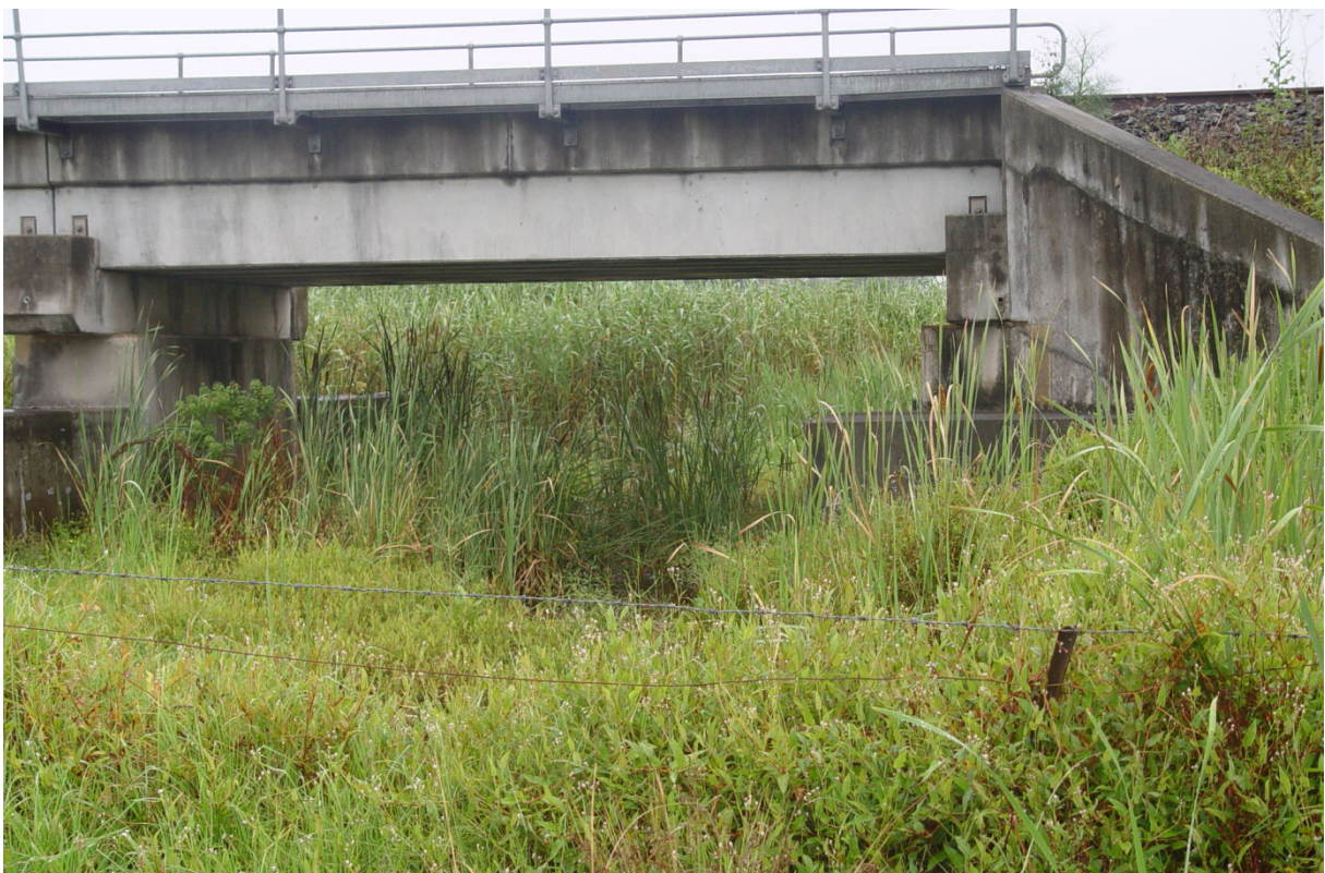
Figure 25: Heavy weed infestation at waterway crossing 3, looking upstream.
