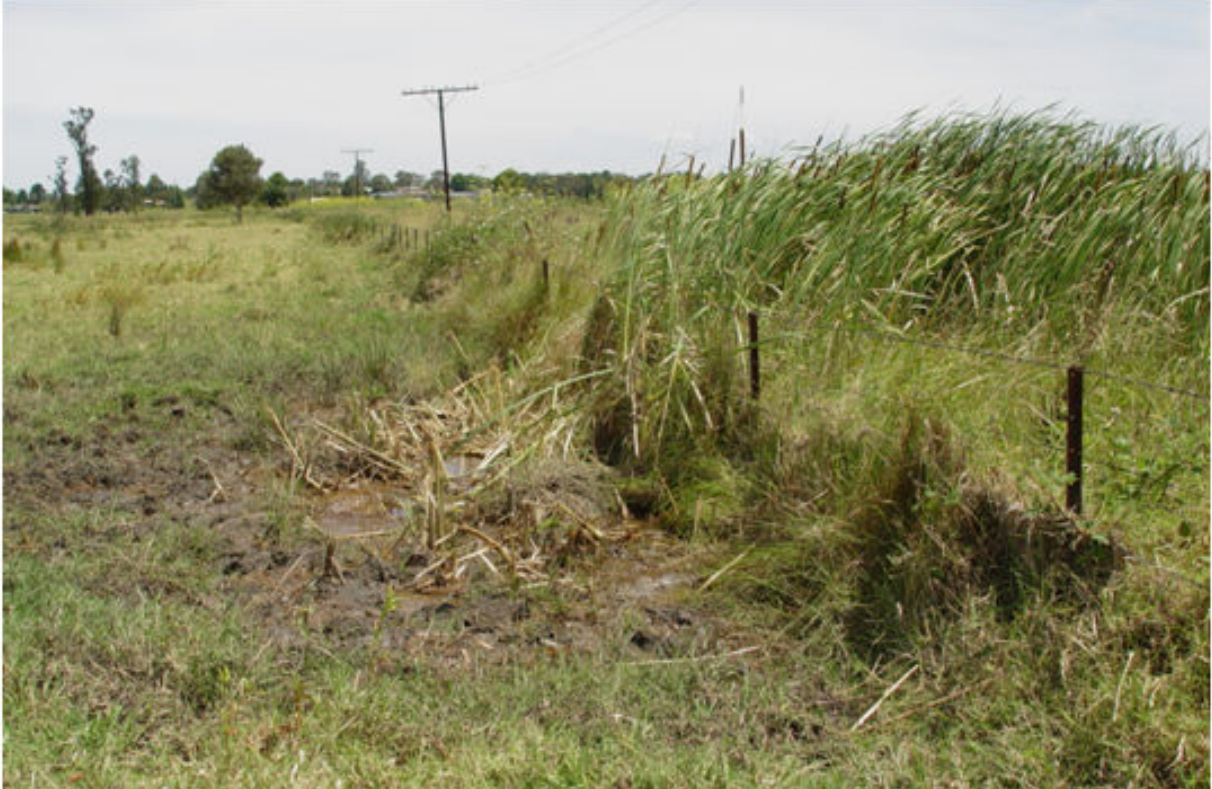
Figure 8: Low lying wet area at intermediate culvert between waterway 1 and waterway 2
