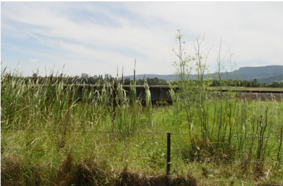
Figure 9: Intermediate Culvert at low lying area between waterway crossing 1 and waterway crossing 2
