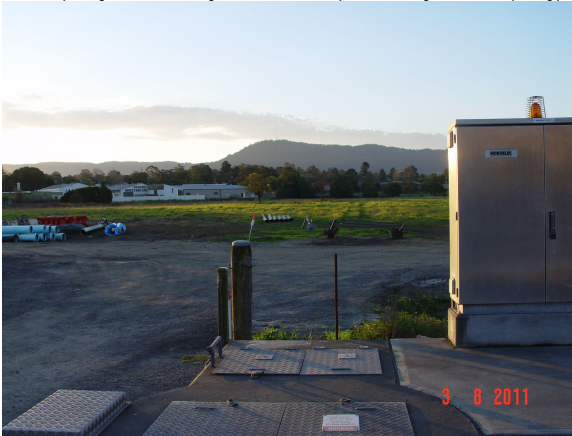
Photo 64- Sewer pump station on Shoalhaven Starches land, with location of proposed gas main route and pressure reduction station in background
