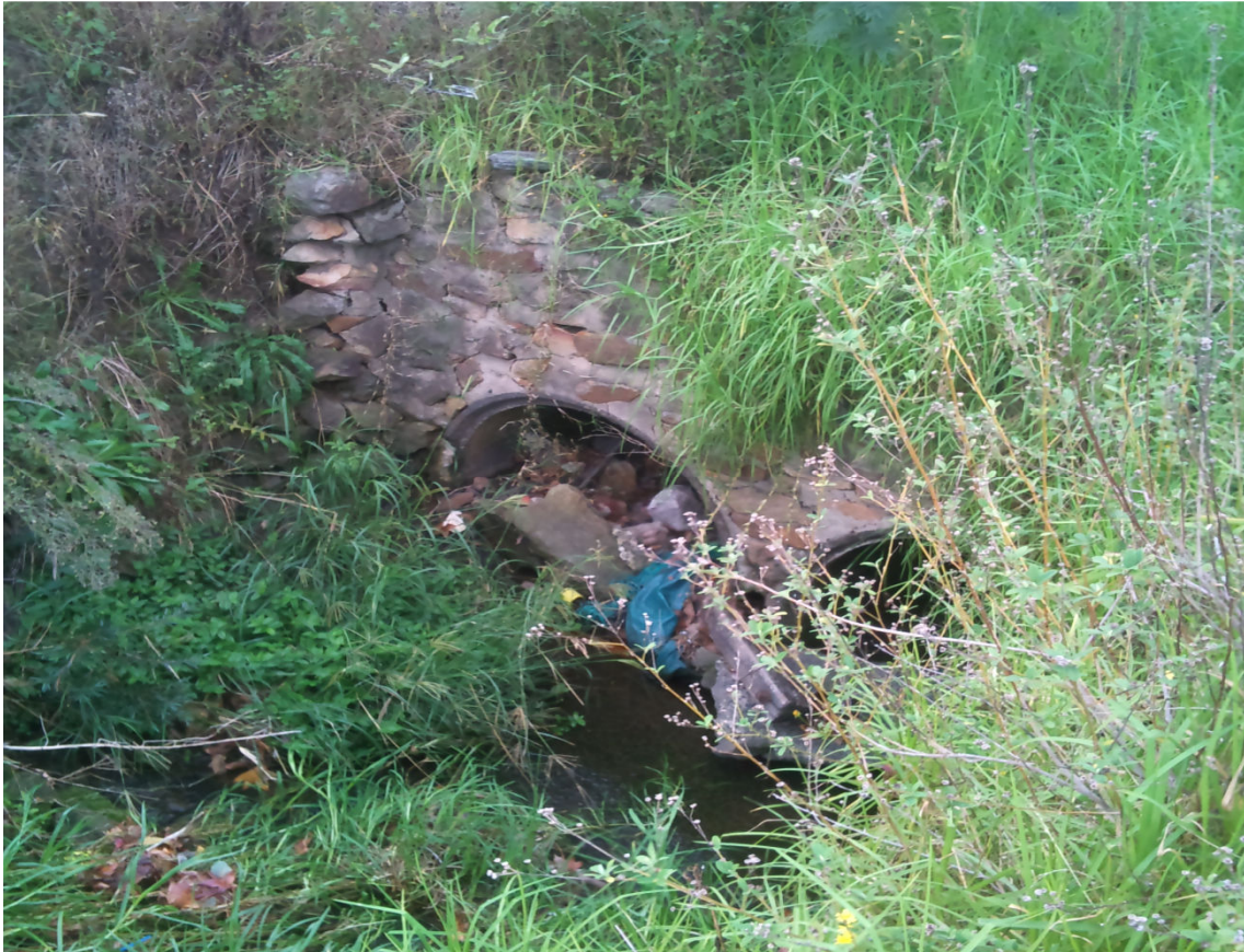
Photo 57- Culvert and support for sewer pipe accross open channel drain in lot 1 DP825808
