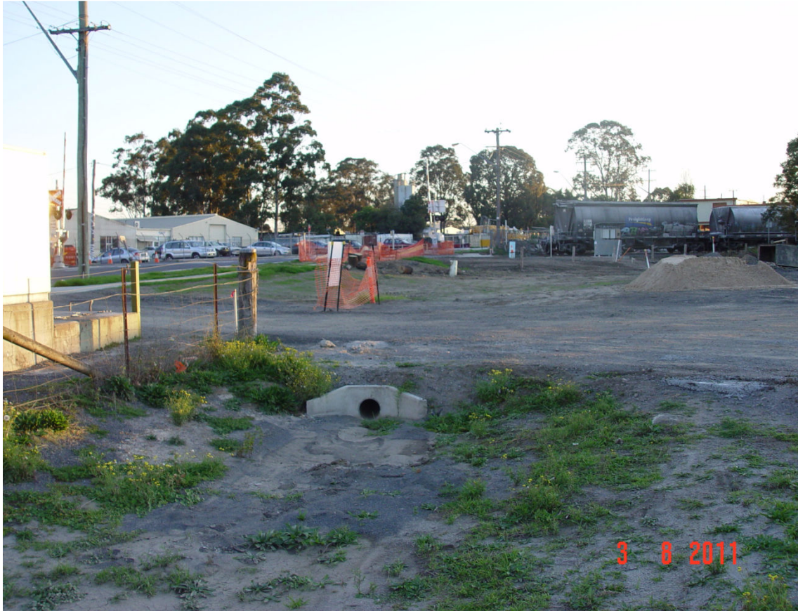
Photo 65- Civil works at most likely position of proposed gas main crossing of Bolong Road
