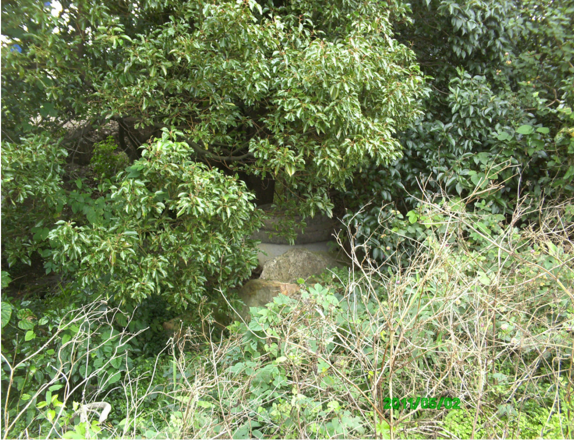
Photo 59- Sewer man hole in open drain along north boundary of Lot1 DP 825808
