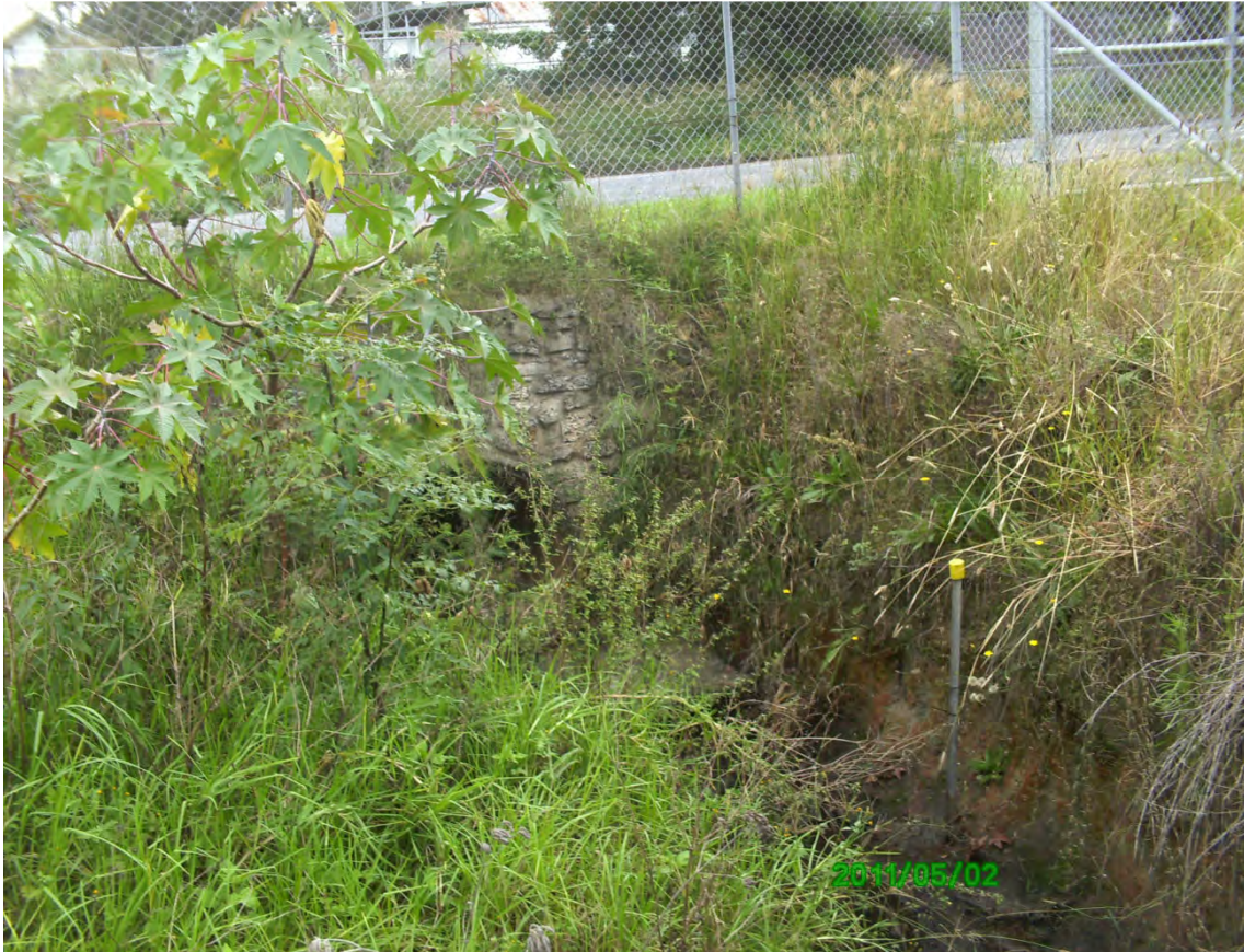
Photo 55- Headwall and culvert under Railway Street, at direction change of proposed gas main
