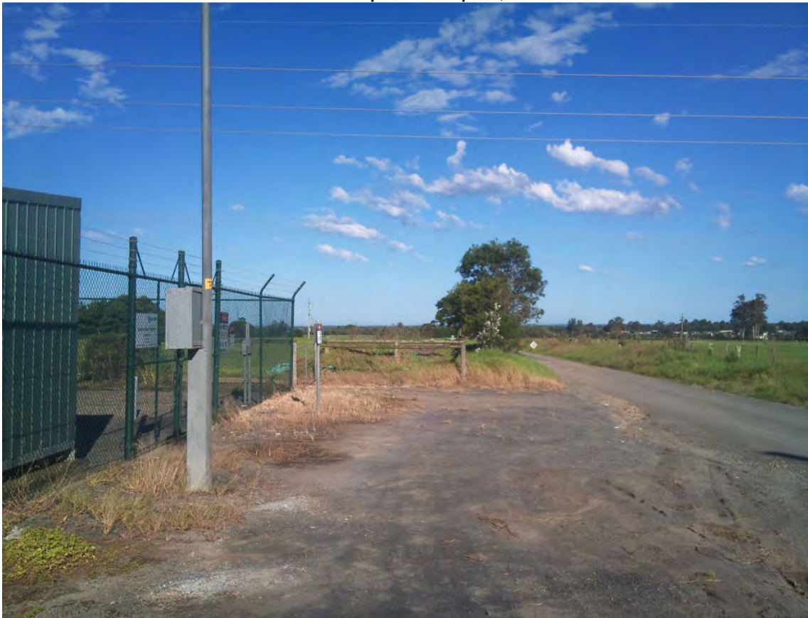
Photo 2 Pestells Lane Eastern Gas Pipeline tie-in point for existing ActewAGL gas pipeline
