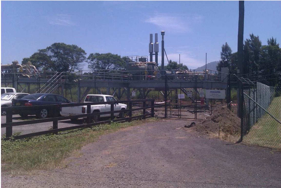
PHOTOGRAPH 4-1 ACTEWAGL GAS HEATER
