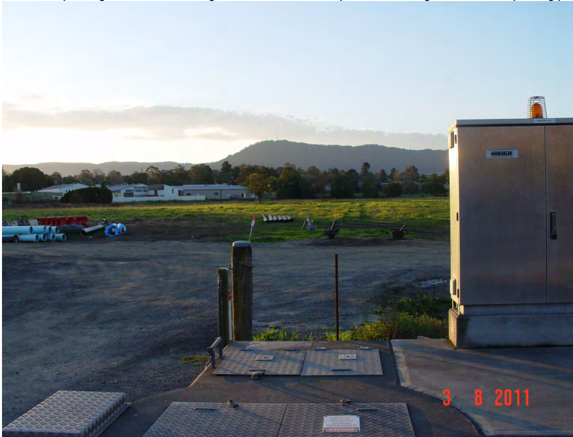
Photo 64- Sewer pump station on Shoalhaven Starches land, with location of proposed gas main route and pressure reduction station in background
