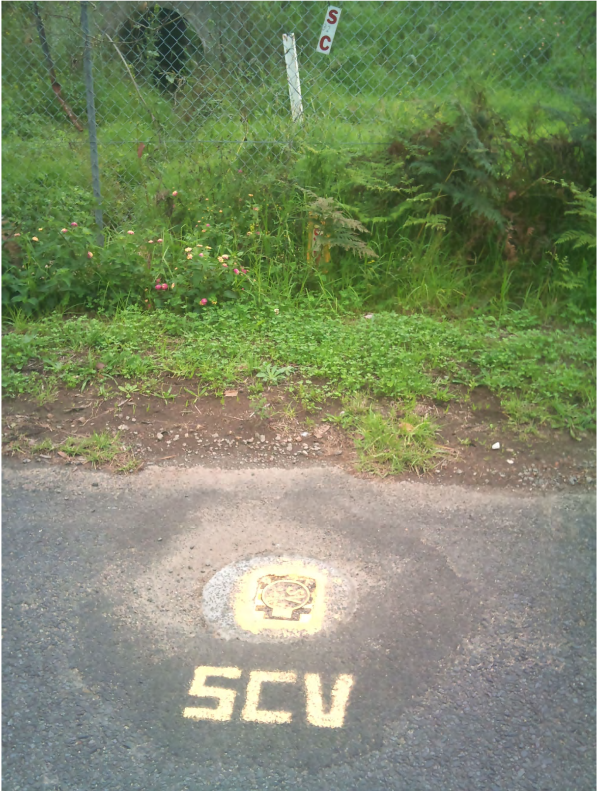
Photo 46- Scour valve in Railway Street
