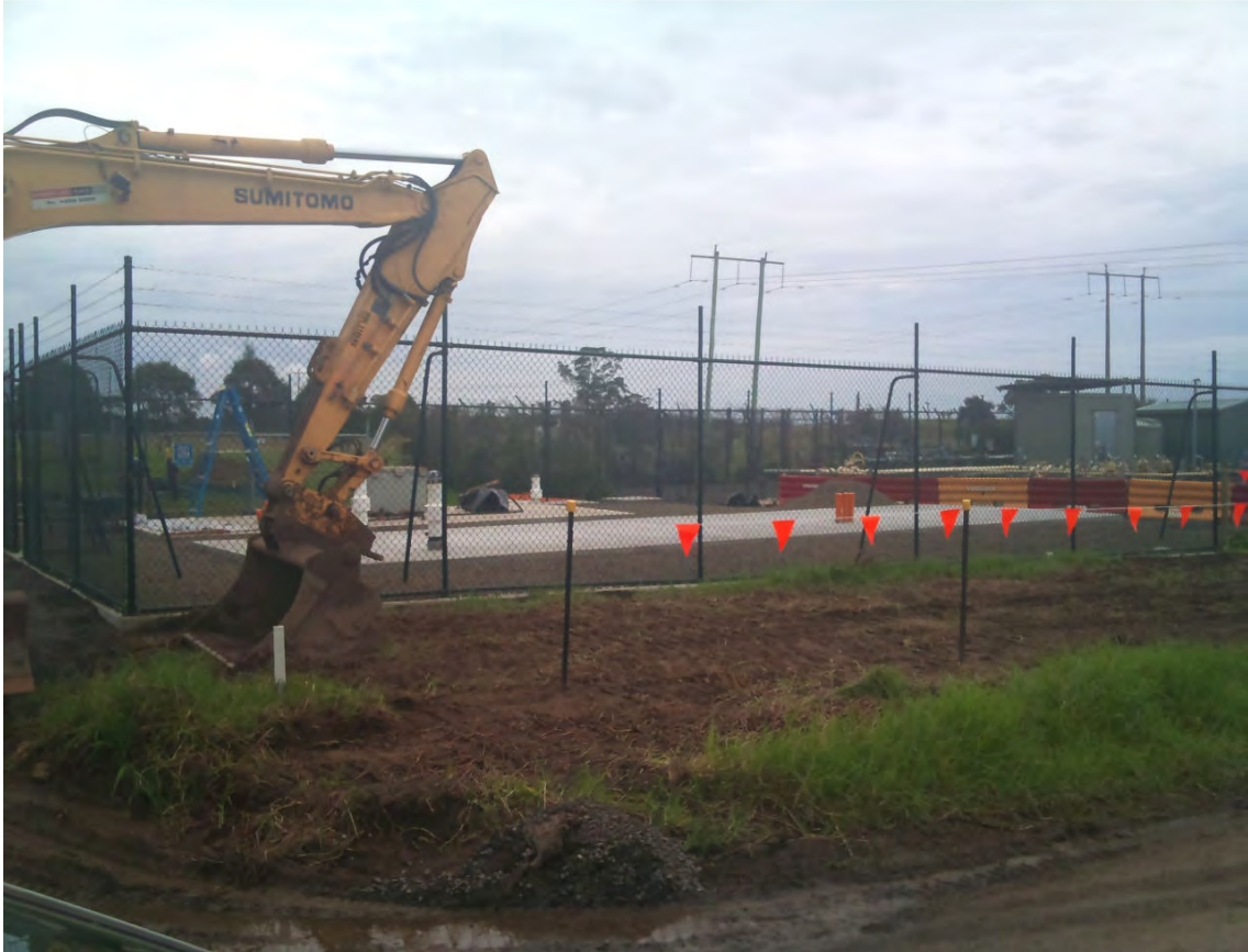
Photo 1-Pestells Lane Eastern Gas Pipeline tie-in point, with valve and meter station
