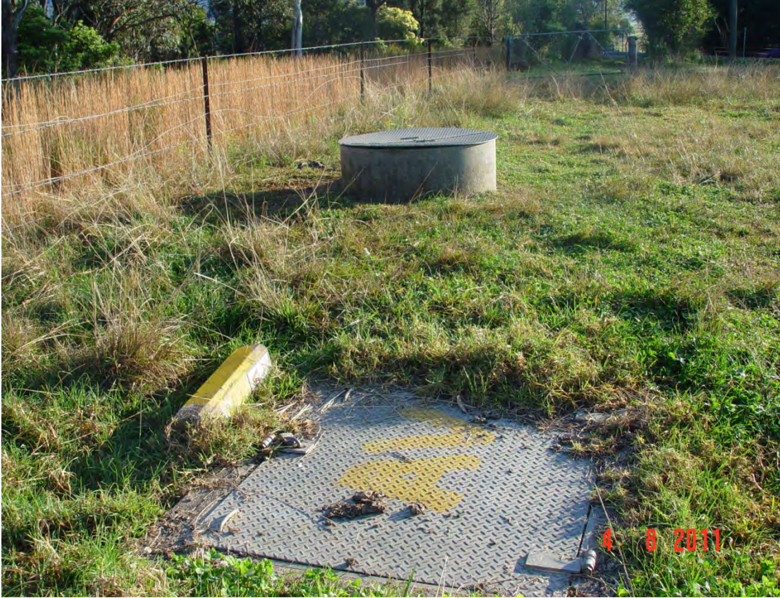
Photo 33- Water main infrastructure in un-named road reserve
