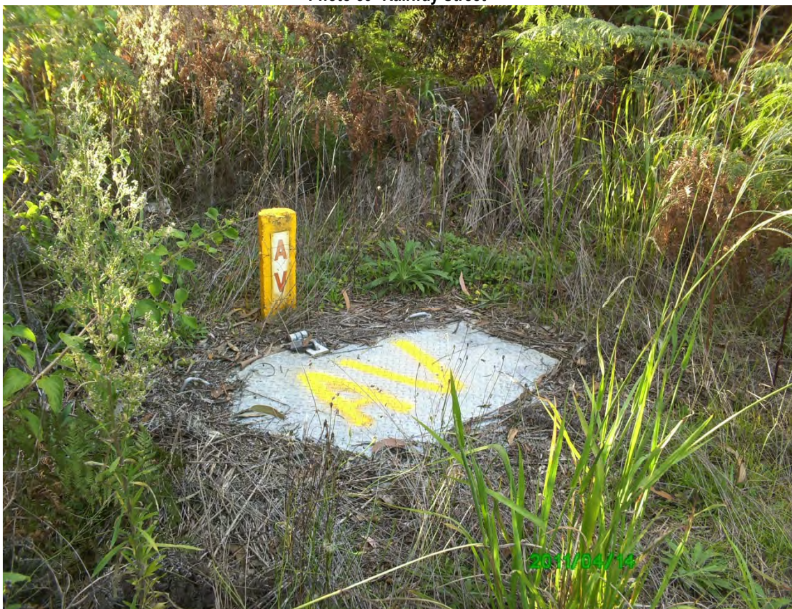
Photo 40- Water main infrastructure in Railway Street road reserve
